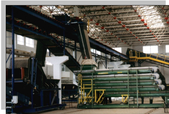
composting plant Beijing, composting hall
